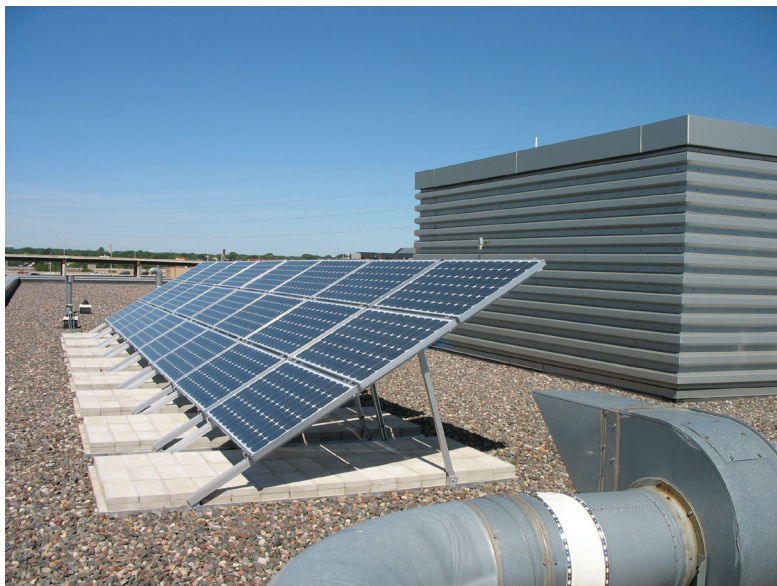
The Currie Maintenance Facility's solar array is one of three owned by the City of Minneapolis. The three photovoltaic systems produced 12,500 kWh of electricity last year.
