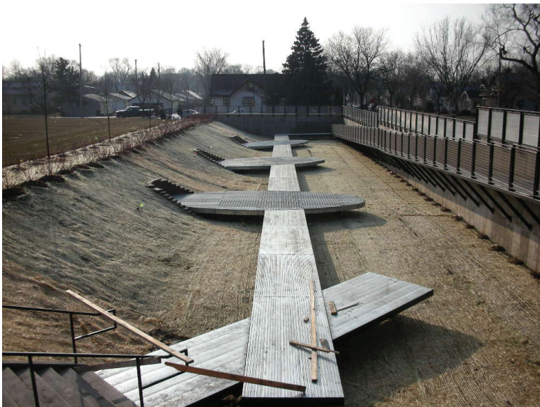
Folwell School Interpretive Rain Gardens (under construction) This project removed nearly two acres of asphalt and boosted the school’s environmental curriculum. Students will use the rain garden walkway to learn about managing stormwater.
